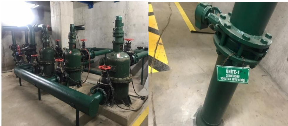
Figure 4.4. Penstock and Butterfly Valves.
