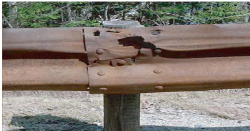
Figure 3.6. Steel beam guardrail deformation [77].
