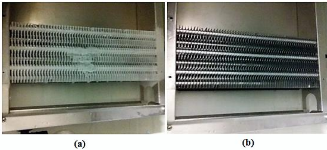
Figure 5.8. Evaporator (a) before defrosting and (b) after defrosting.
