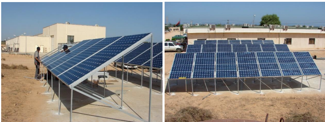
Figure 3.1. Solar panels in Libya.
