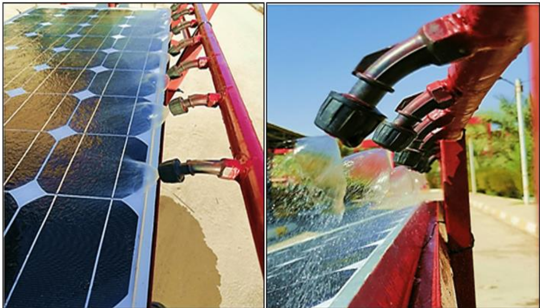
Figure 3.5 Upper water nozzle spraying.
