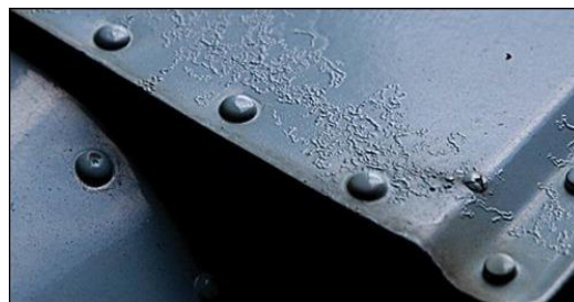
Figure 2.5. Filiform corrosion of Mg alloys [50].
