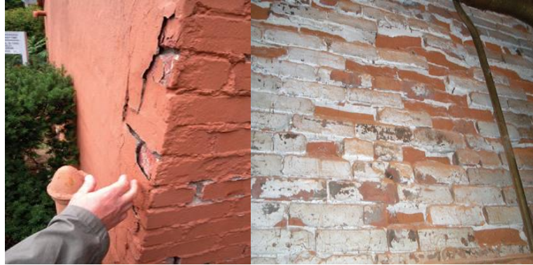
Figure 2.10. Damage of bricks is caused by the migration of soluble salt through them [68].
