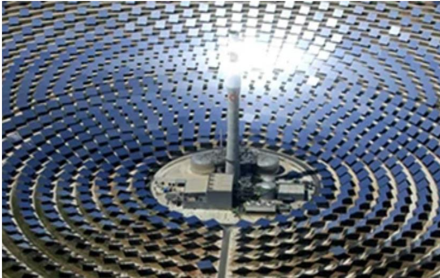
Figure 3.2. Concentrated solar power project. Nur Energie/Tunisia [82].
