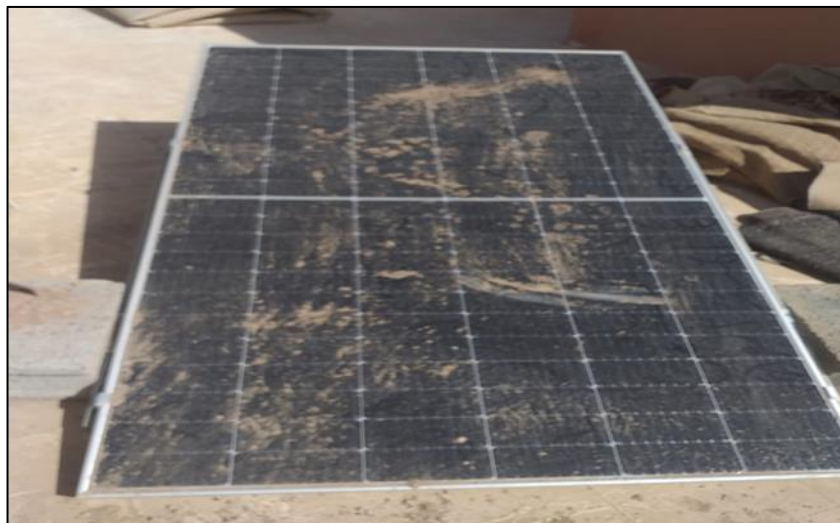
Figure 4.4. A small amount of dust deposits on the solar cell surface.
