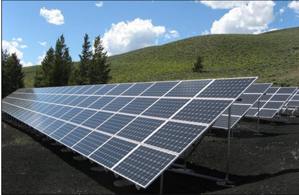
Figure 1.1. A solar cell system in generating electric power [8].
