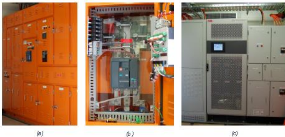
Figure 6.2. (a) An alternating current switch panel, (b) Automatically activated circuit breakers, (c) Bi-directional Inverter.
