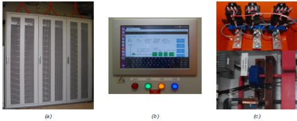
Figure 6.3. (a) The three-rack battery system, (b) The controller system HMI screen local , (c) Voltage and current transducers.
