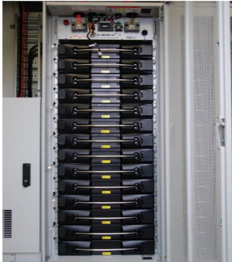
Figure 6.15. One rack of the LG Lithium-Ion battery container with 14 power slots.
