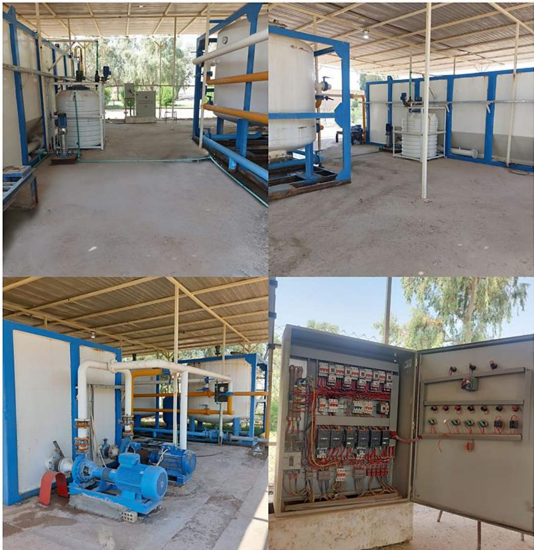
Figure 3.1. A Picture of the Station Before Adding PLC.
