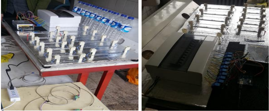
Figure 5. 8. Electrical load panel with control unit
