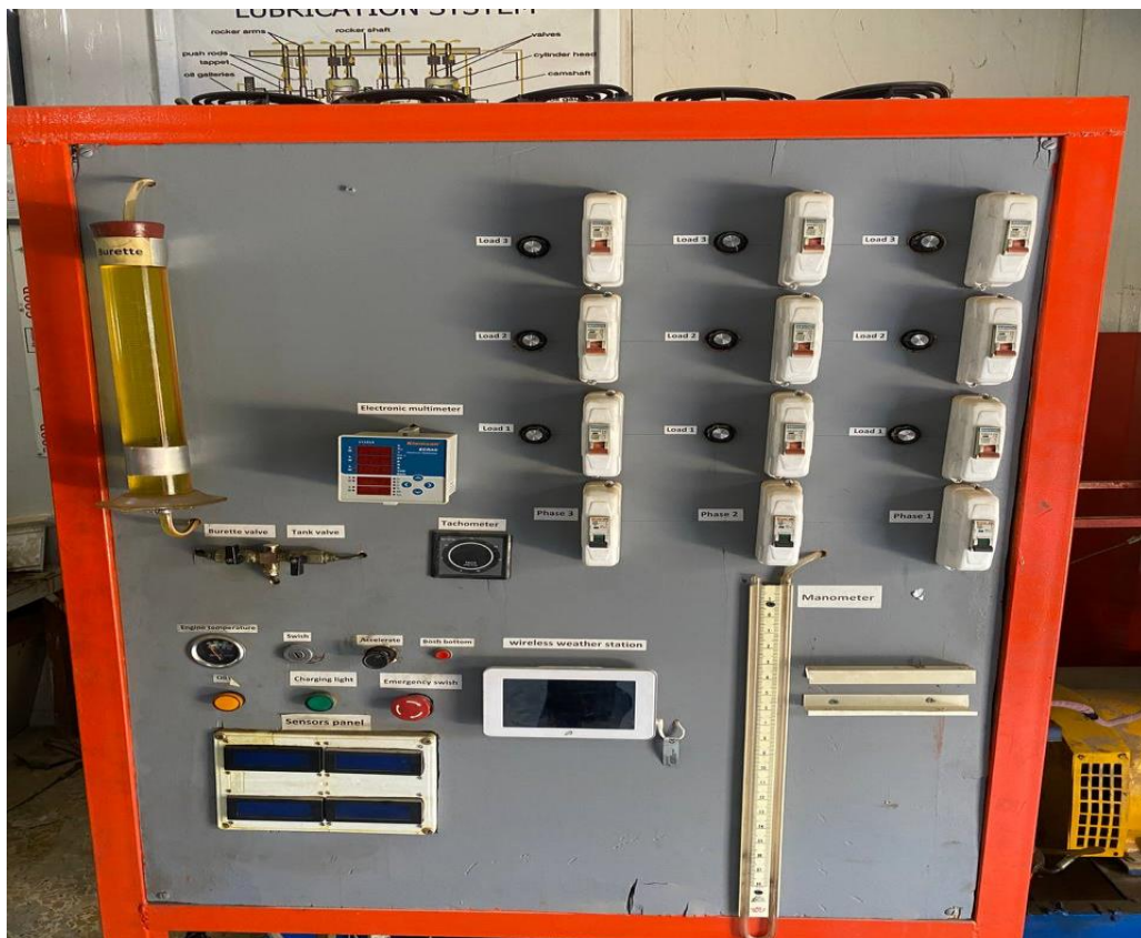
Figure 3.4. Control panel and measurement.
