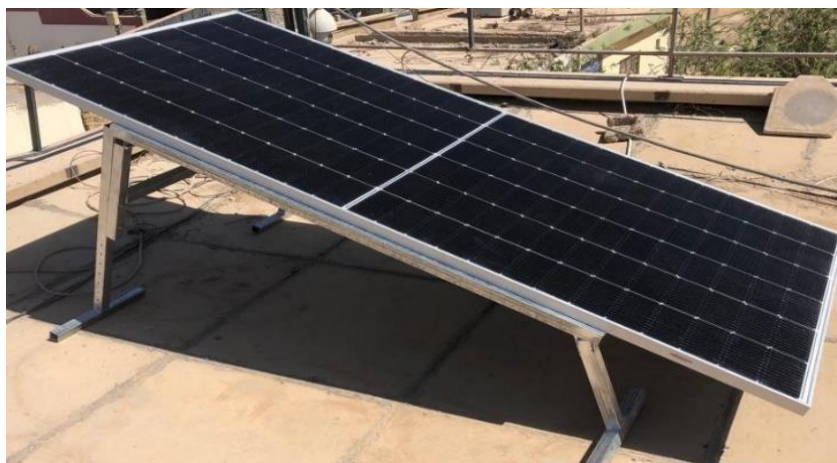
Figure 4.5. Photovoltaic panel, nominal power 580 W.
