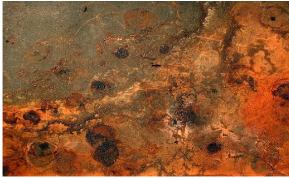
Figure 3 1. Rust the most familiar example of corrosion
