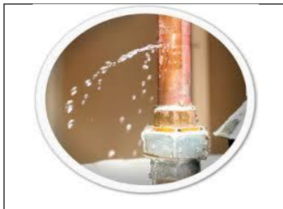
Figure 3. 3. A pinhole leak in a copper pipe caused by corrosion[11].
