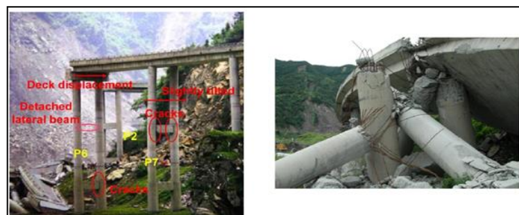
Figure 11. Possible failure mechanism of Baihua Bridge and collapse of the bent 5 [10]
