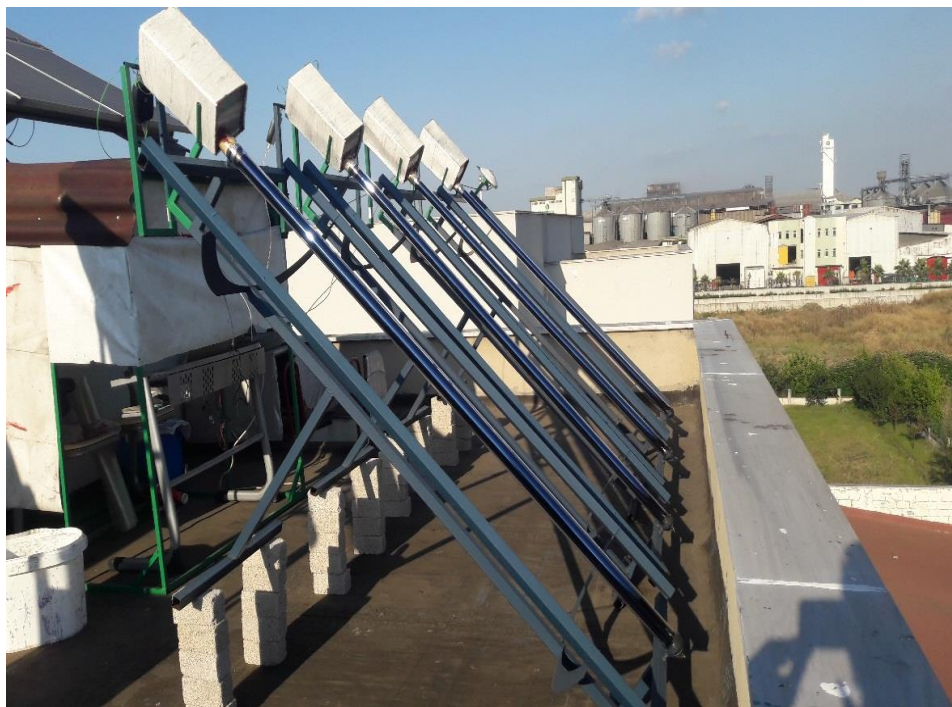
Figure 3.9. Photograph showing the heat pipes receives solar radiation at an angle of 56°.
