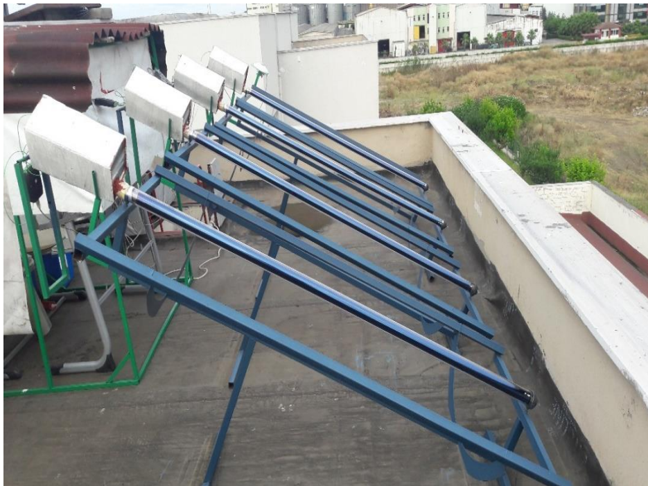
Figure 3.7. Photograph showing the heat pipes receives solar radiation at an angle of 26^\circ .
