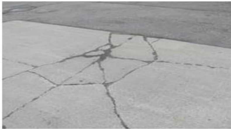
Figure 3.26. Punch-out failures in rigid pavements [60].
