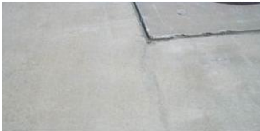
Figure 3.23. Shrinkage cracking in pavements [60].
