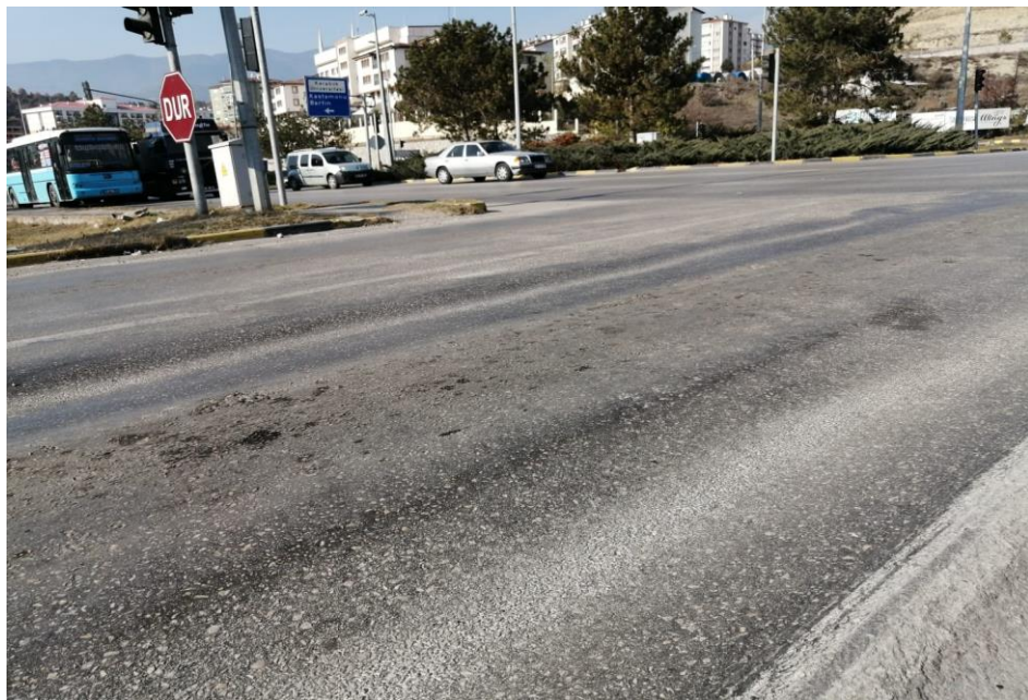
Figure 5.1. Asphalt rutting and deformations in Karabük – Turkey.
