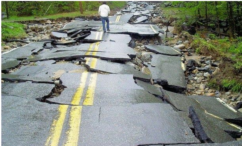
Figure 4.1. Deformation due to environmental factors [42].
