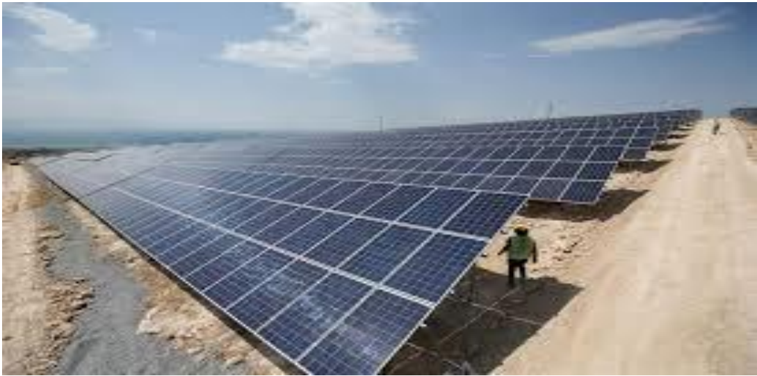
Fig. 1.4 Solar Power plant
