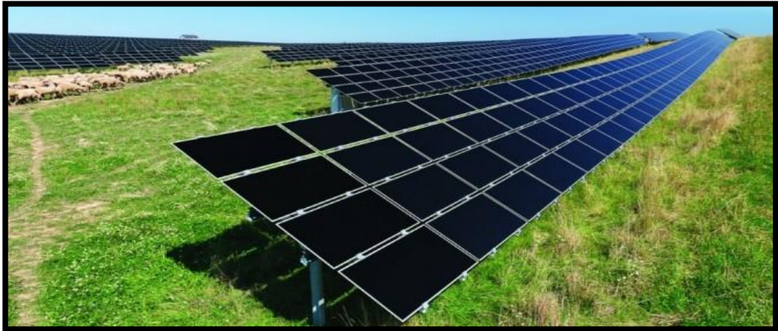
Şekil 2.6. İnce film panel kullanılan sistem ( https://energyinformative.org , 2020).
